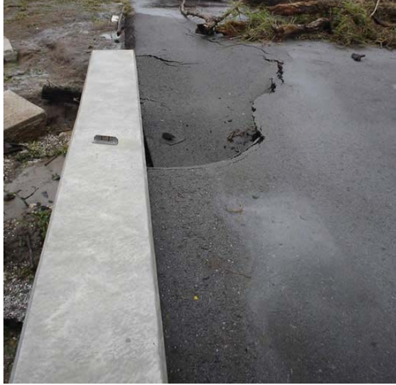
Figure 6: Example of Light Damage from Damaged-Passable Category
