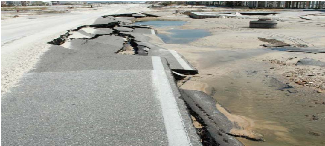
Figure 7: Example of Medium-Damage Severity from Damaged-Passable Category
