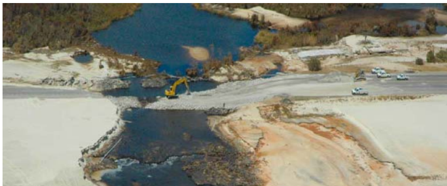
Figure 11: Example of Impassable Damage
