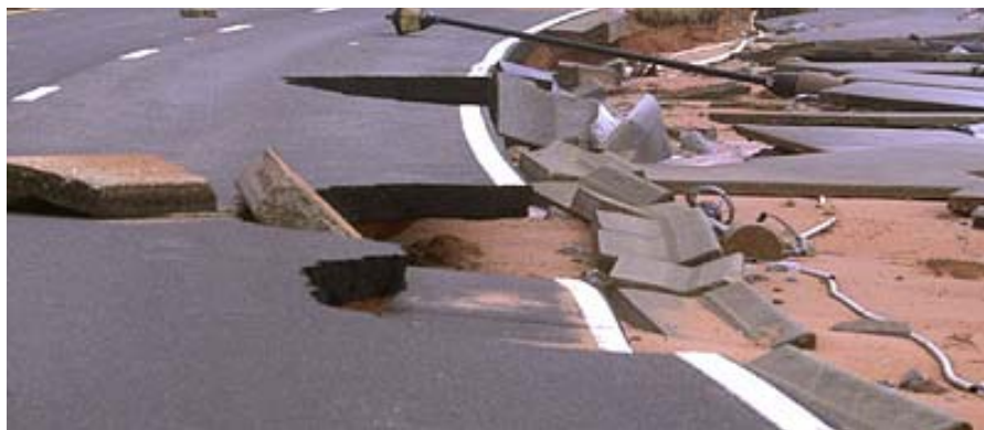
Figure 9: Example of Medium-Damage from Damaged-Dangerous Category
