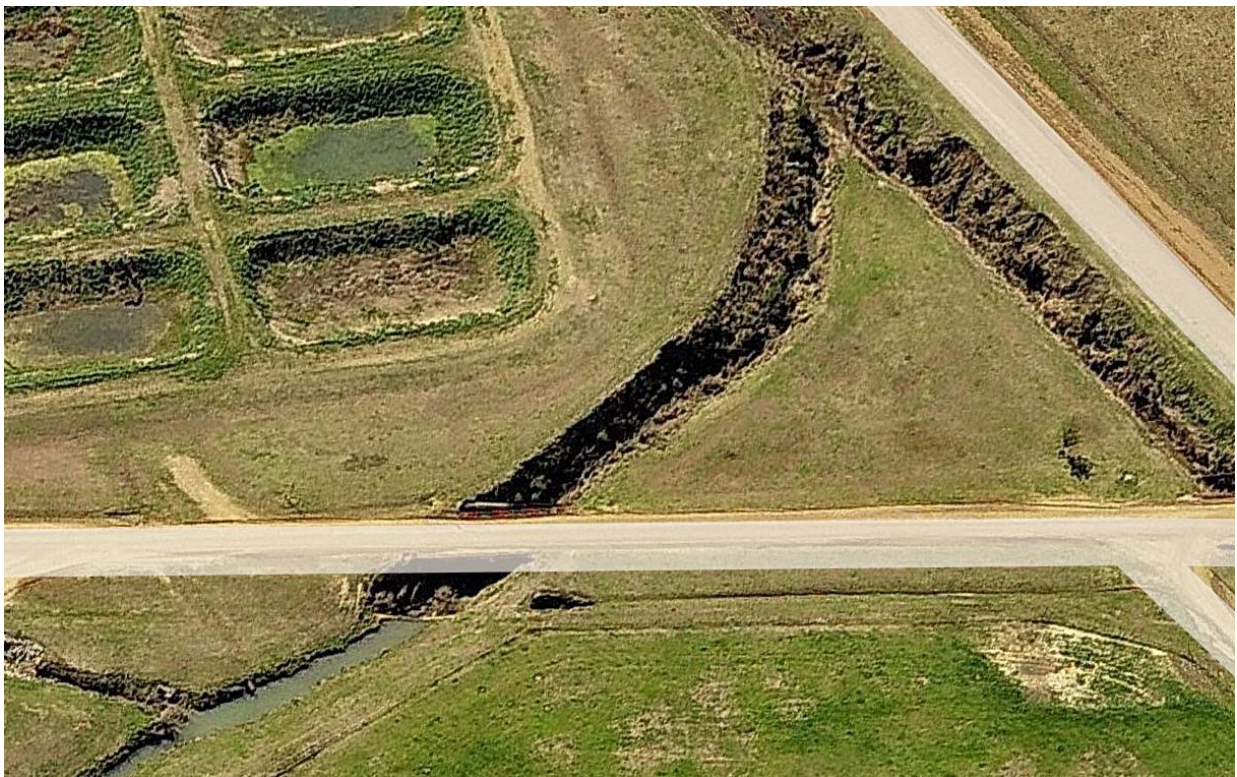
Stream Bank Instability Downstream of a Dam on a Catalpa Creek Tributary (Images from Bing.com)
