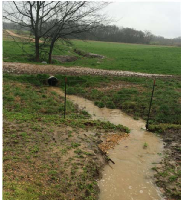
Site 7c NRCS Practice 410 – Grade Stabilization Structure (Drop Pipe-Riser)
