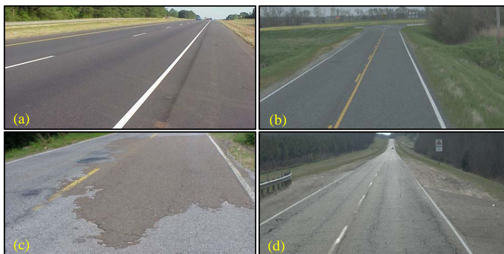
Figure 1. Pavement Conditions: (a) very good, (b) fair, (c) poor, and (d) very poor.
