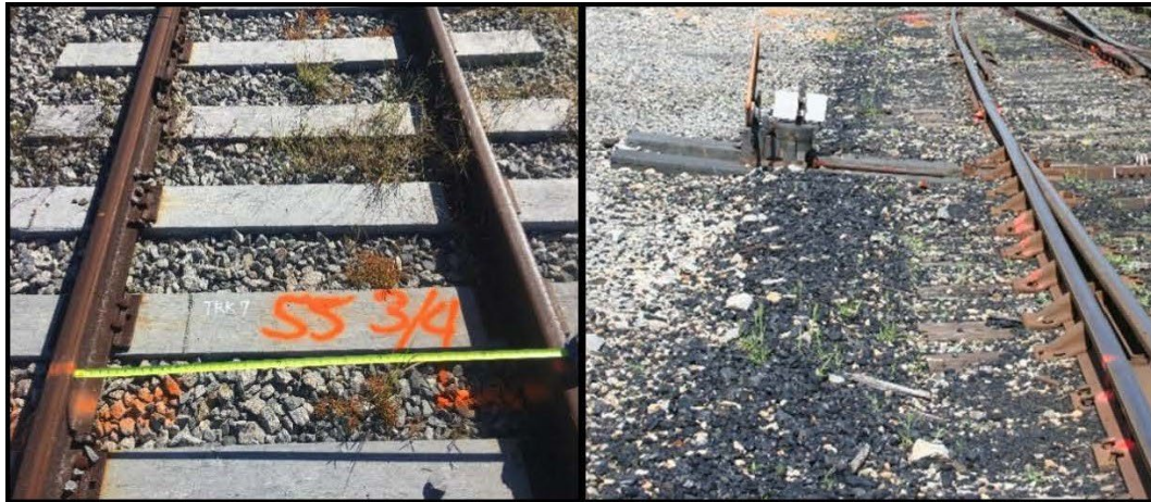
(a) Thermal effects cause tight gage
