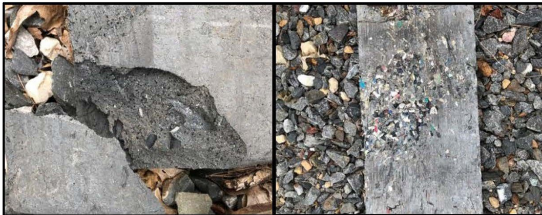
(c) Installation damage
